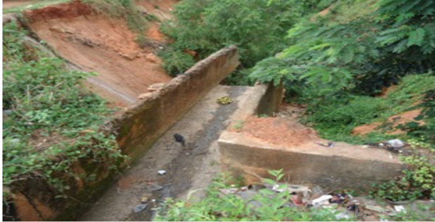
Plate 3: Inconclusive remediation effort at OFGES
