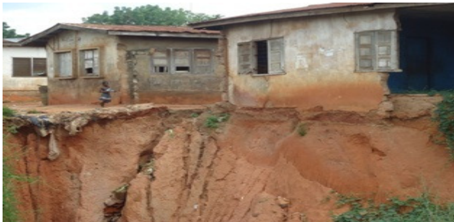
Plate 2: Houses threatened by gully erosion within OFGES
